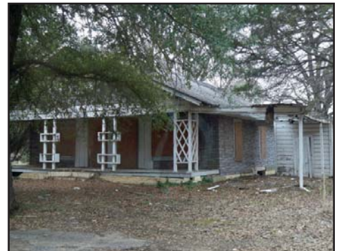
Example of structure on property, dilapidated
